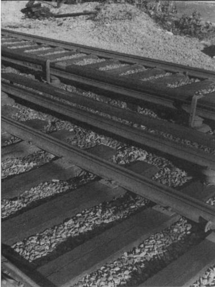
650 volts dc. "Chairs" mounted on extra-long ties support third rail. (Author photo)
